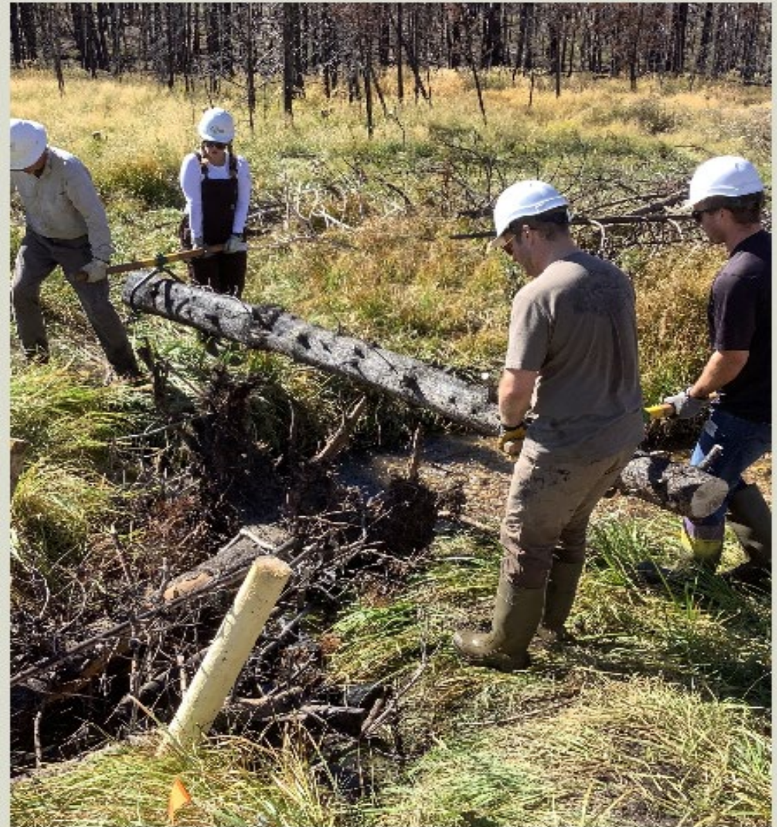
Volunteers work to install a post-assisted log structure (PALS). PALS provide opportunity for sediment storage behind the structures while promoting floodplain connectivity, additional wood recruitment, and riparian health.
