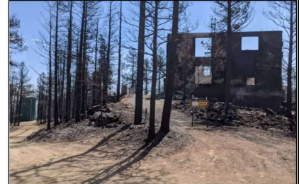
Burned Water Treatment Plant, NM
